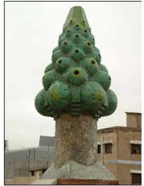
Gaudí populated the roof of the Palau Güell with a variety of imaginative chimneys.
